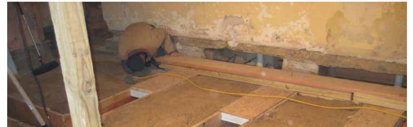
Wall excavated with needle beams- the gaps were filled with concrete to provide a continuous footing.
