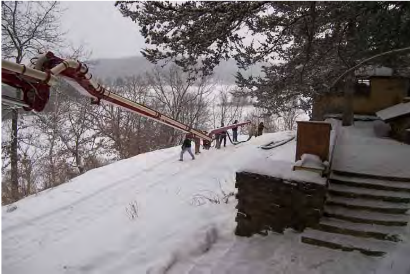
A concrete pumping truck is used to deliver concrete into the Guest Wing.
