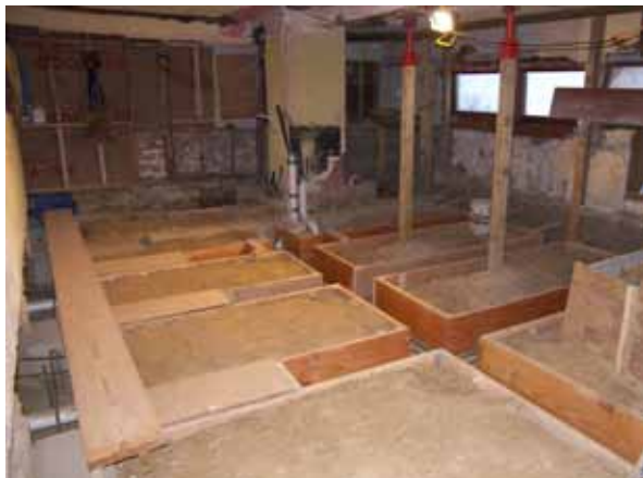
Same room as above with trenches completed, these were poured continuously using a concrete pump truck.
