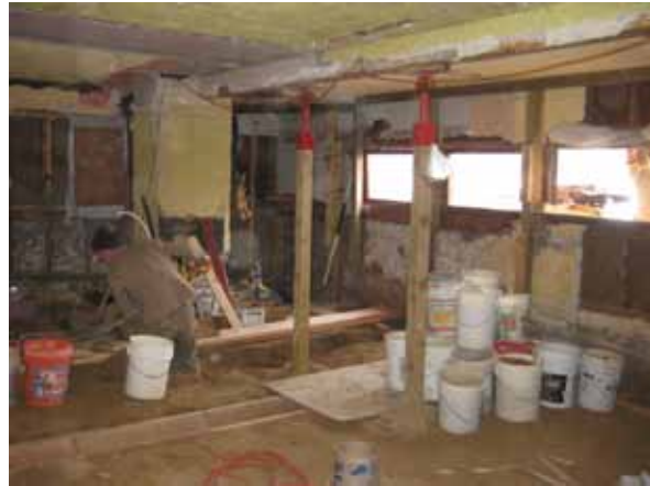
Room #5, located underneath the Living Room, team members had to hand dig grade beam trenches and move earth out with 5 gallon buckets.
