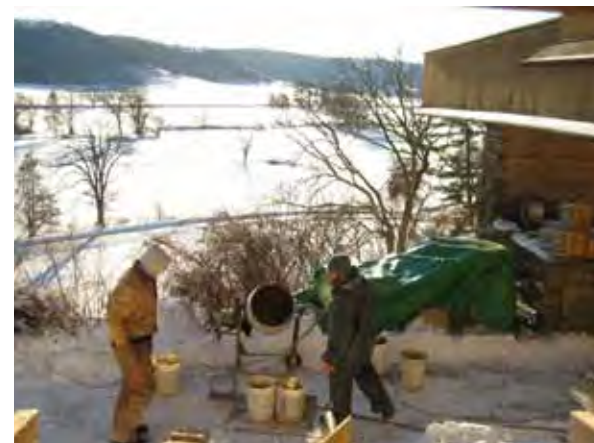
Hand mixing was necessary so that as sections underneath walls were excavated they could be filled.
