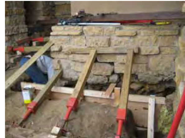
One of the stone walls that is failing due to lateral forces.
